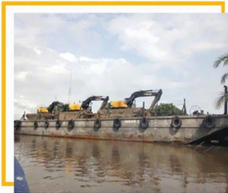
Swamp Excavators on Board Ramp Barge at Ovhor Field for capital Location Dredging
